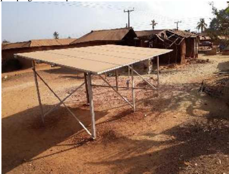
Figure 1: Picture of the solar part of the borehole in Kotaa
